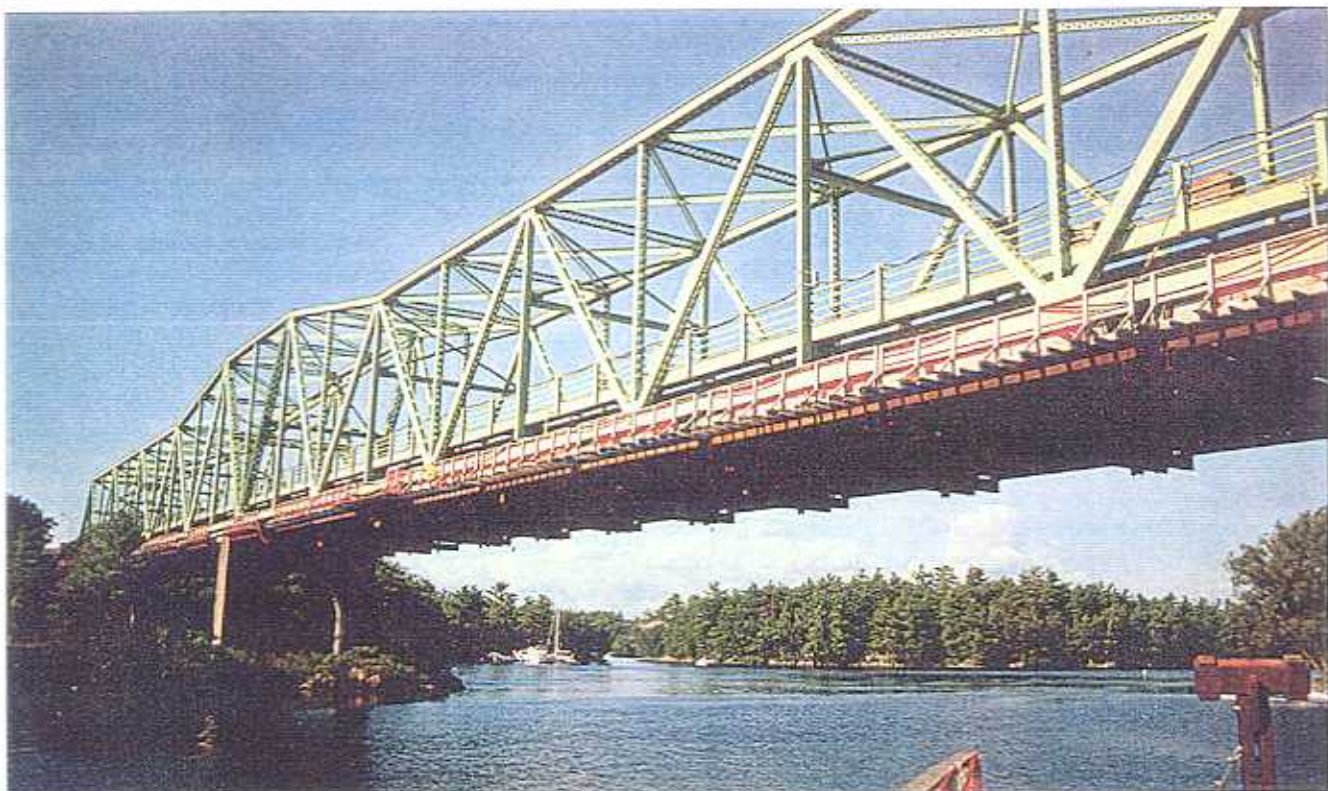
TRUSS MEMBERS PREVENTED CONTINUATION OF A MAINTENANCE WALKWAY ALONG THE SPAN'S EAST SIDE, AND FORCED USE OF AN OVERHEAD GANTRY SYSTEM TO MEET TRUCK CLEARANCE LIMITS. A RUBBER-TIRE-MOUNTED CRANE HANDLED DECK SECTIONS UNREACHABLE BY EITHER GANTRY SYSTEM.
