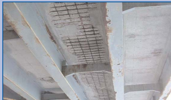
View of bridge deterioration
