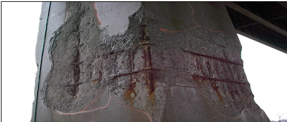
Figure 3: Typical spalls on south column of pier W17
