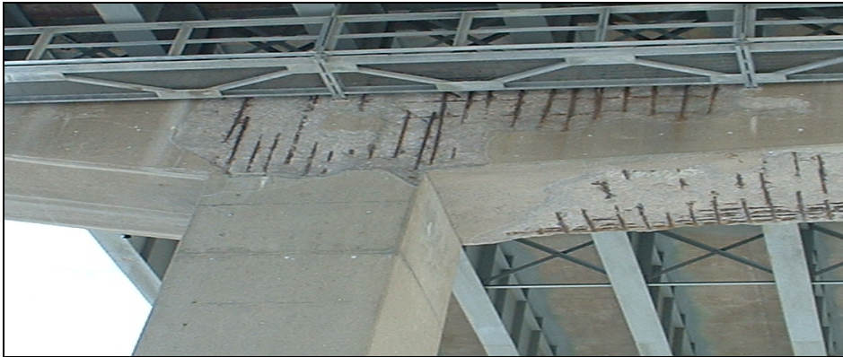
Figure 2: Typical spalls on pier cap of pier W11
