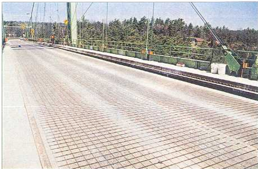
Original deck surface condition on the suspension spans.
