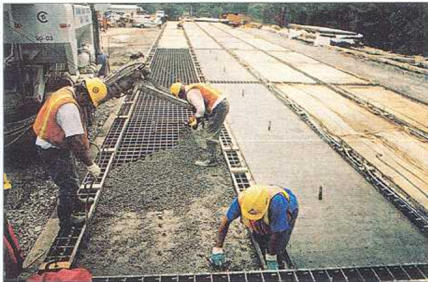
Placing, finishing, and wet-burlap curing of concrete in the deck panels for the Warren-truss spans.
