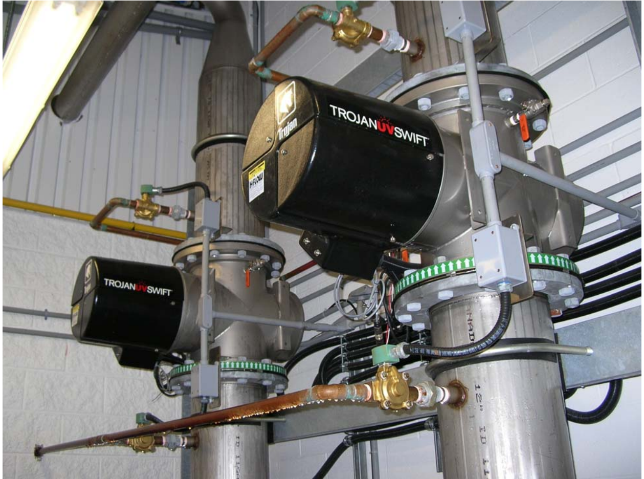
UV disinfection reactors in Cardinal, Ontario
