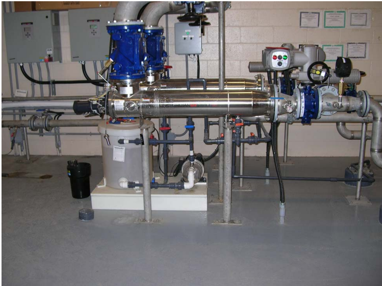
Ultraviolet (UV) disinfection reactors with a chemical clean in place system at Havelock, Ontario
